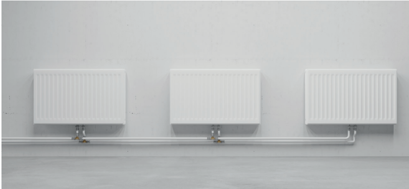
Fig. 47: Double pipe radiator heating.
